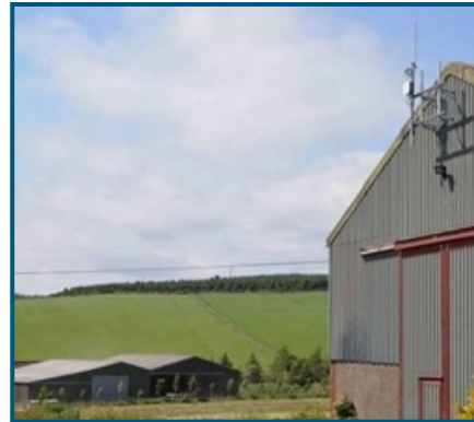
Example of wireless infrastructure installed on farm buildings
